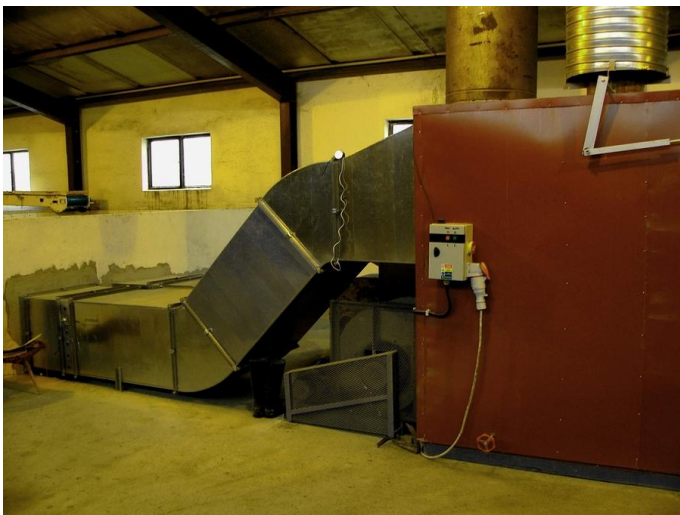
Figure 2. Air-heater for heating of drying medium
