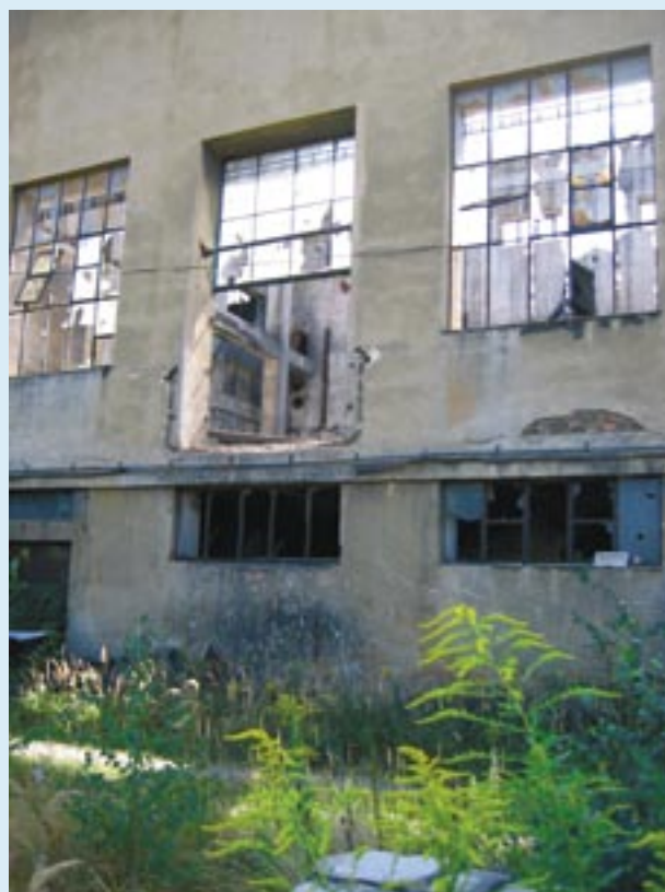
Fig 3.1., 3.2 Sidings of steelwork plant and ancillary buildings in Krakow. Photos: archive IURS, author Y. G. Garb.
