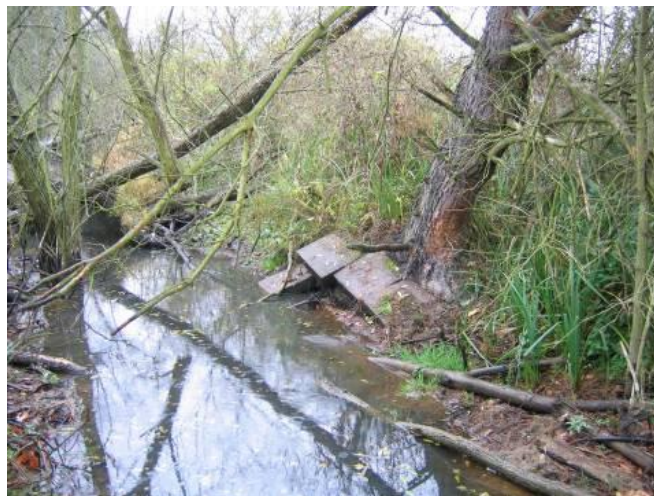
Figure 2 Bank vegetation growing up in the concrete revetment of the riverbed
