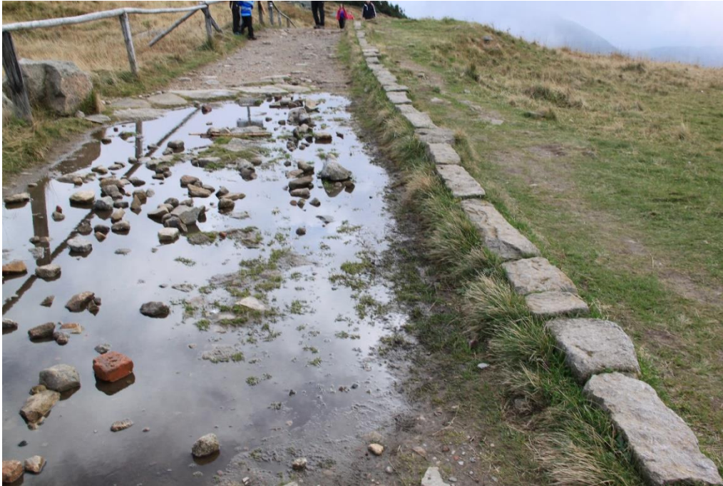
Figure 3 improper drainage of the soil/gravel trail (source: author)
