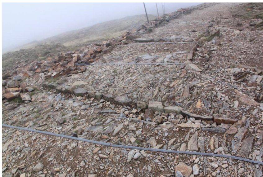
Figure 7 damaged trail with wrongly oriented wedges (source: author)
