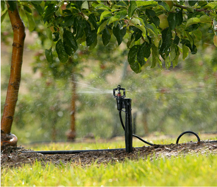
Picture 62 Micro-sprinkler delivers water to plants and influences air temperature and relative humidity (tiirrigation.com)
